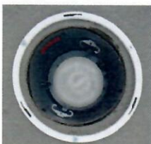
Recessed Light Fixture with the trim and baffle removed. Mounting ring attached to the ceiling and centered.
